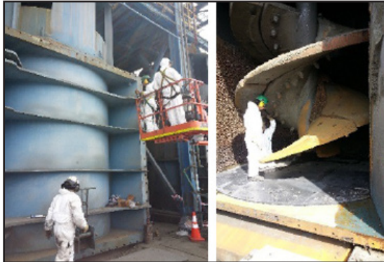
Vertical grinding mill.
