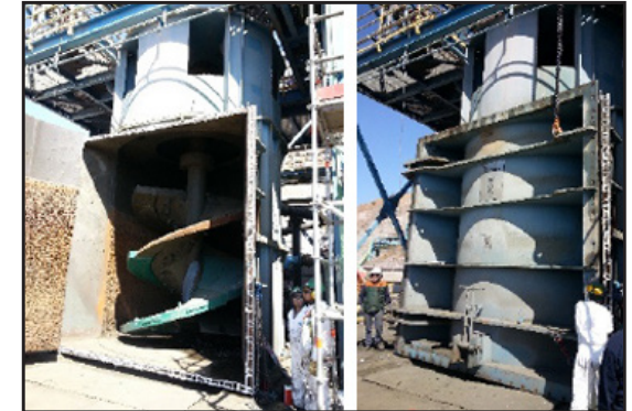
Grinder door closed after applying 860 MPG.
